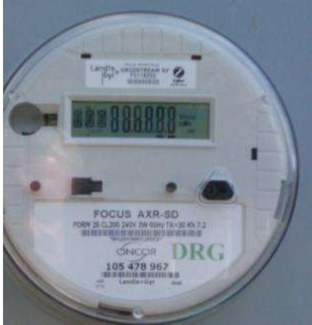
5. Closeup – Main service meter (meter make, model, kWh-out readouts, and meter # visible)
