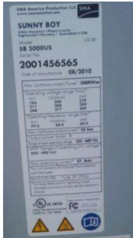
4. Closeup – Inverter specs label
