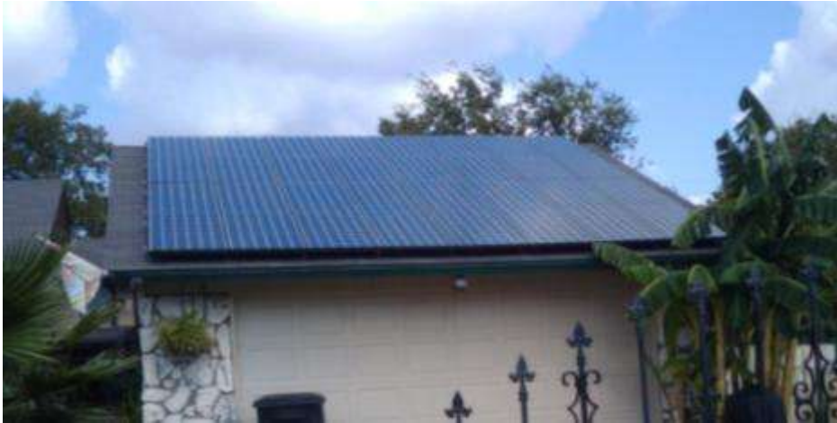
1. Overview – PV array (all modules are visible, countable)
