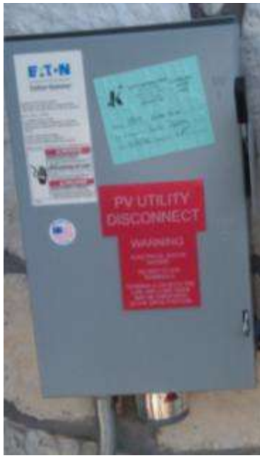
7. Closeup – Utility AC disconnect (shows disconnect type, safety labeling)
